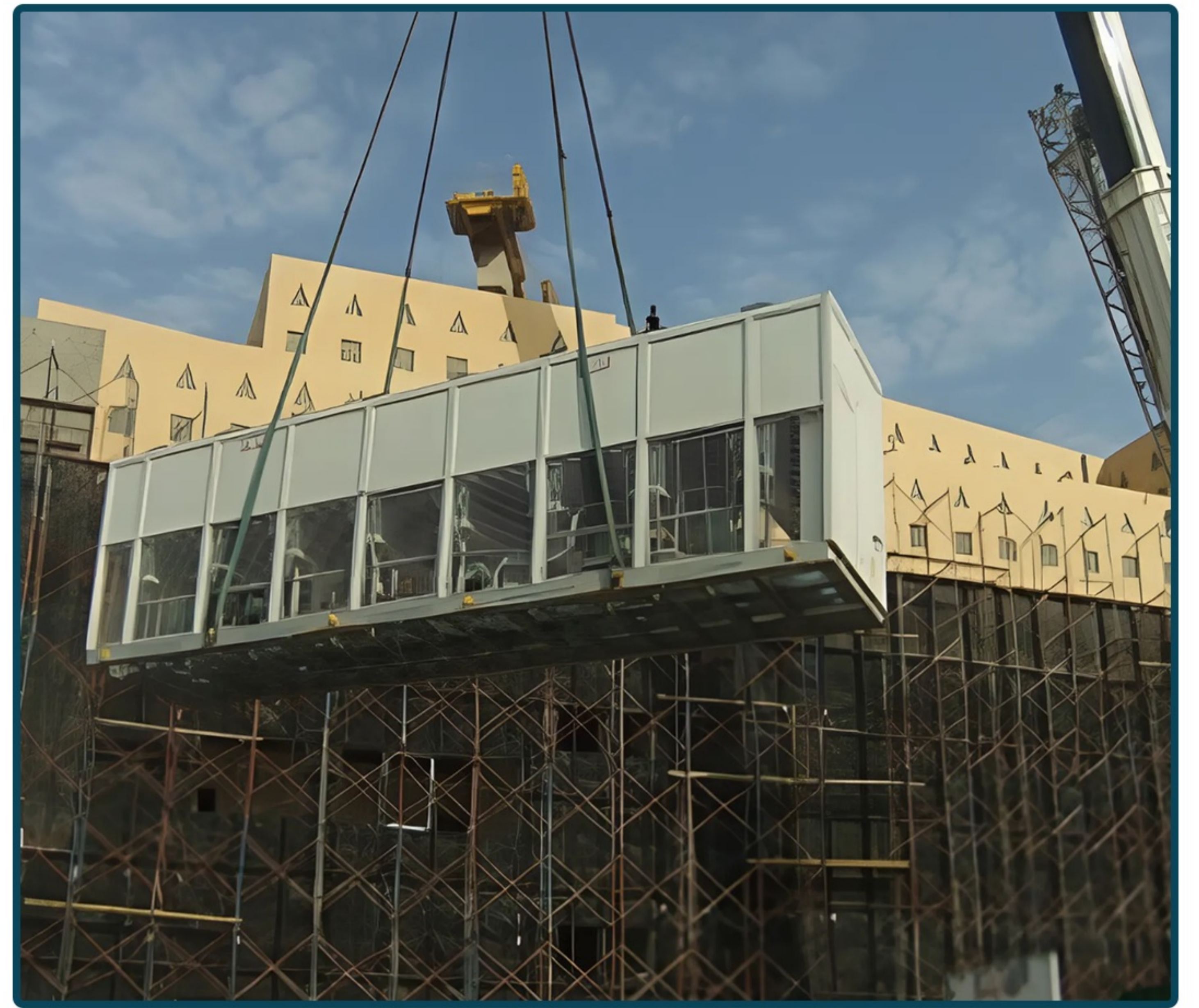
Chiller unit (Air Cooled)
