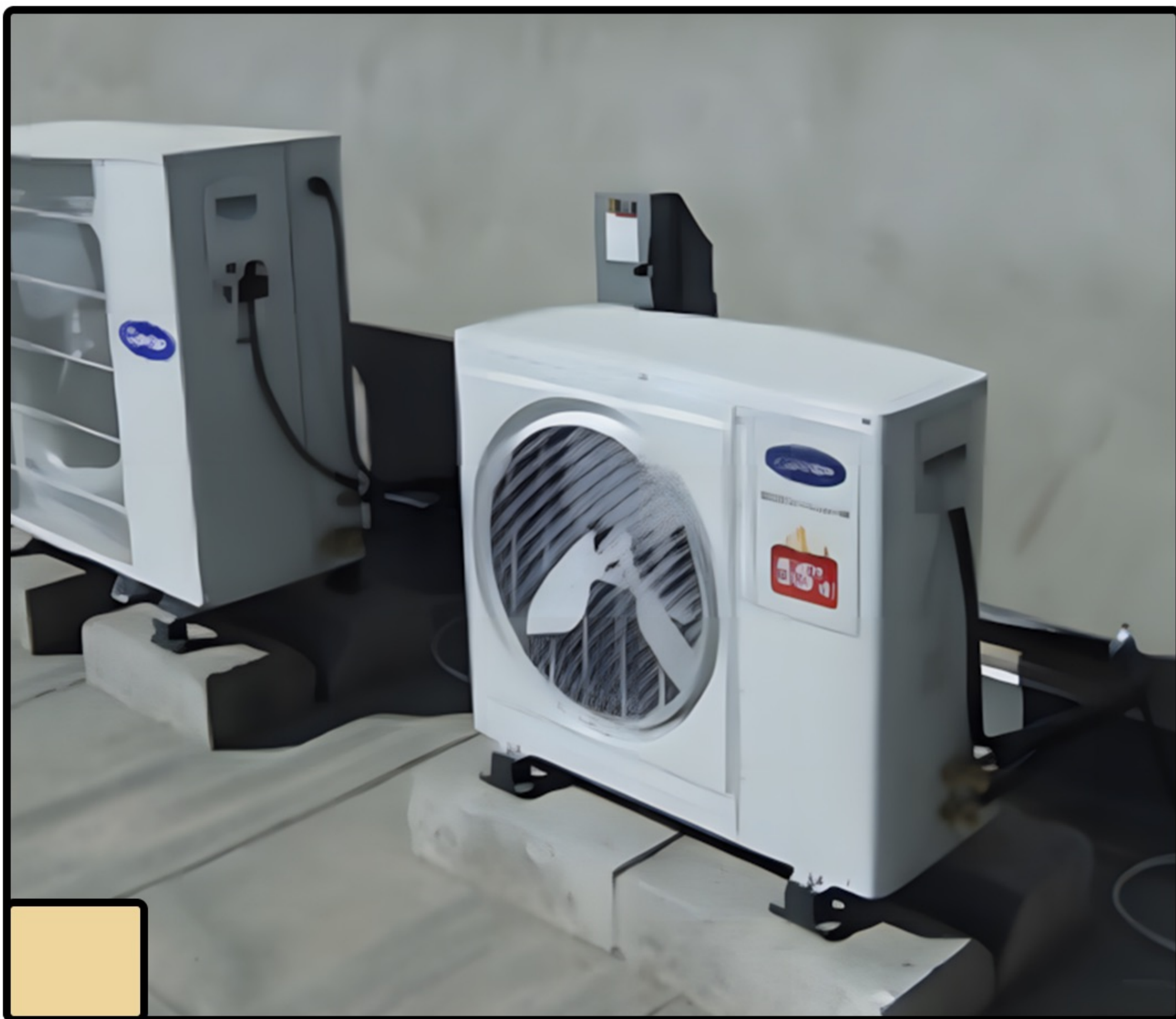
Split unit ( outdoor unit )
